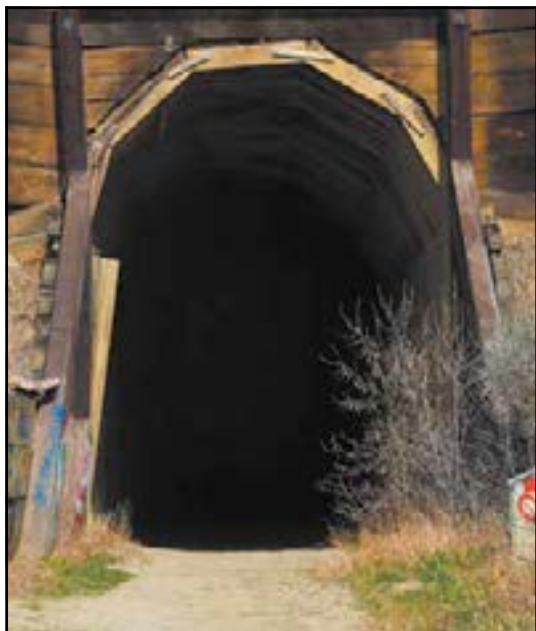
The entrance to the historic Cartwright Tunnel at the end of the Fairview Lift Bridge.
