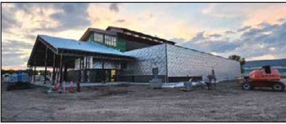
This drone photo shows the new Event Center addition on the right side of the old one and the new sidewalk to the left.
