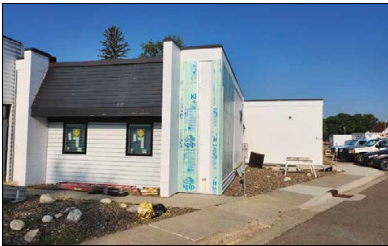
Necessary repairs to the Savage School progressed this summer with B&B Builders as the contractor. (Photo submitted by Savage School)
