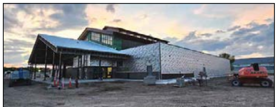
This drone photo shows the new Event Center addition on the right side of the old one and the new sidewalk to the left.
