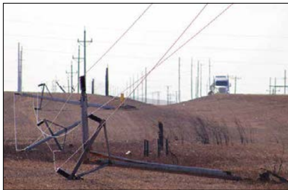
A burned power pole sits off 109th Avenue, between Ray and Tioga, N.D., after fires came through the area on Oct. 5, 2024. (Jacob Orledge/North Dakota Monitor/ProPublica)
