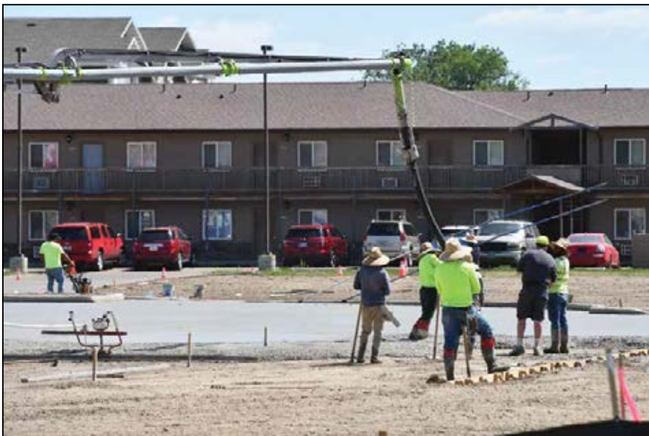
Construction crews pour the concrete foundation and parking for the new Dollar General store on Holly St. in Sidney.
